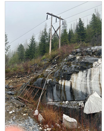
Transmission lines & hydro tower
